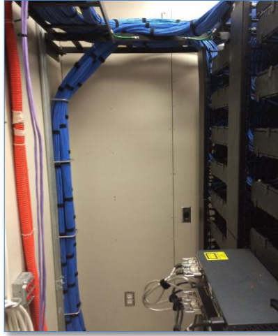
Figure 2—Secured wiring closet on Willow campus is organized and well-kept.
